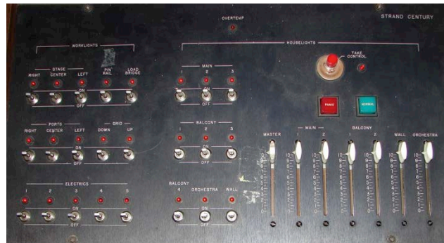
House/Work light panel in Booth
