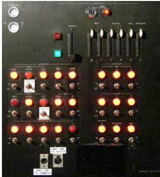
House/Work light panel DSR.
